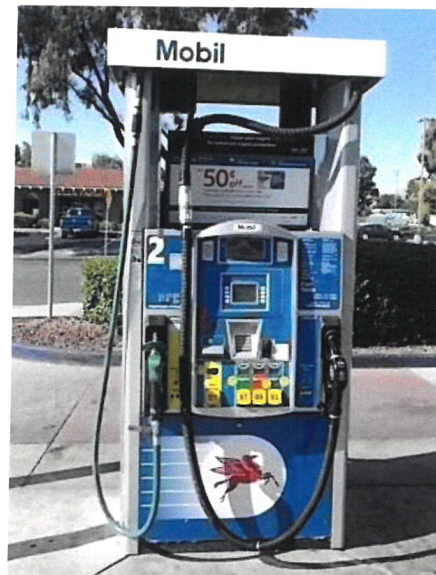
EXISTING - DIESEL PUMP
