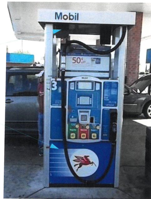
EXISTING - GASOLINE PUMP
