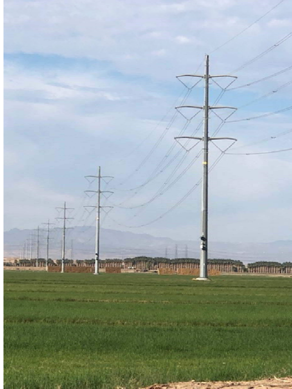
Figure 4: Example Tie-Line Structures
