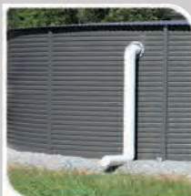
6-Inch Overflow Drainage Pipe
