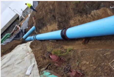
WTP Raw Water
