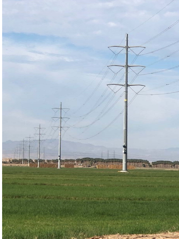
Figure 4: Example Tie-Line Structures
